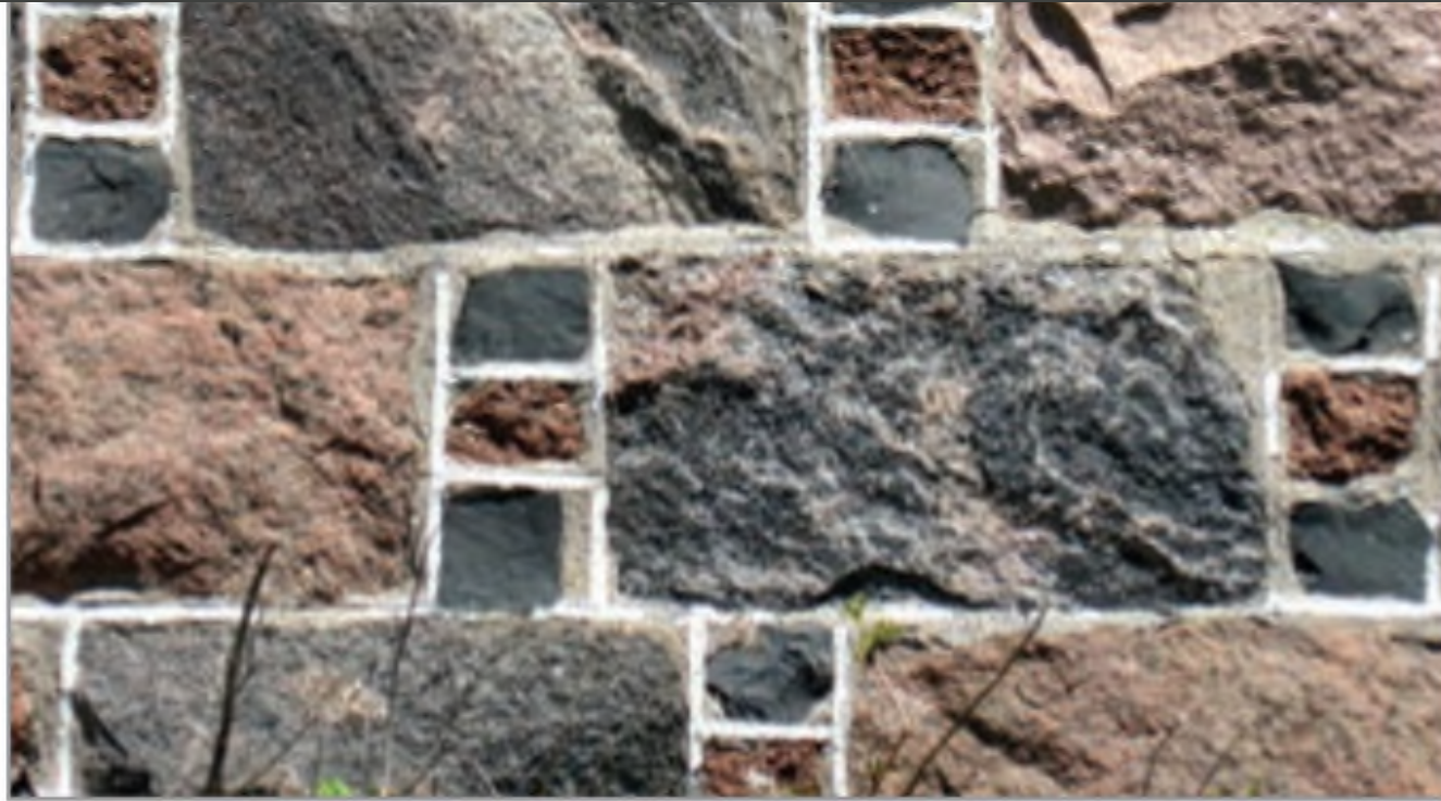
FIG. 16. CRELLIN'S ABERDEEN BOND STYLE MASONRY, WITH 3 SNECKS, MCCORQUODALE HOUSE, I 29 TH LINE, NO. 6565, NEAR HARRINGTON, OXFORD COUNTY. | KAREN E. ARMSTRONG.
